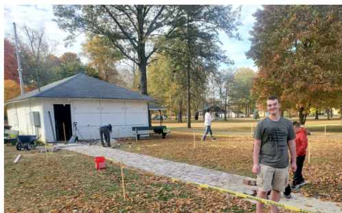
Garret Rose earning his Eagle Scout by installing a new brick walkway to the enclosed shelter at Ivester Park
